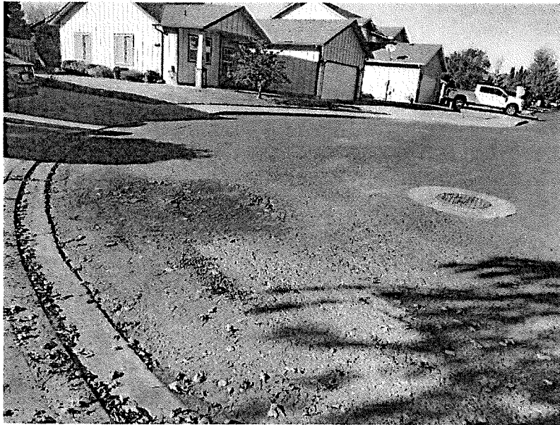
Figure 22: Pavement Condition - S.E. Newgate Court
