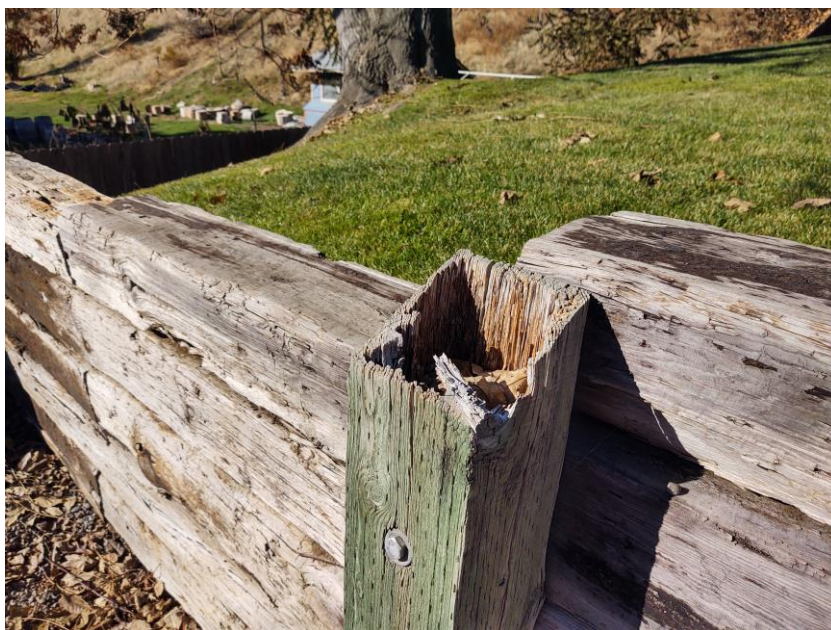
Figure 8: Retaining Wall Post Condition
