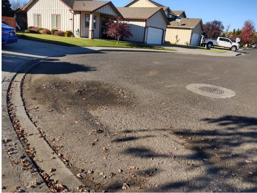
Figure 22: Pavement Condition - S.E. Newgate Court
