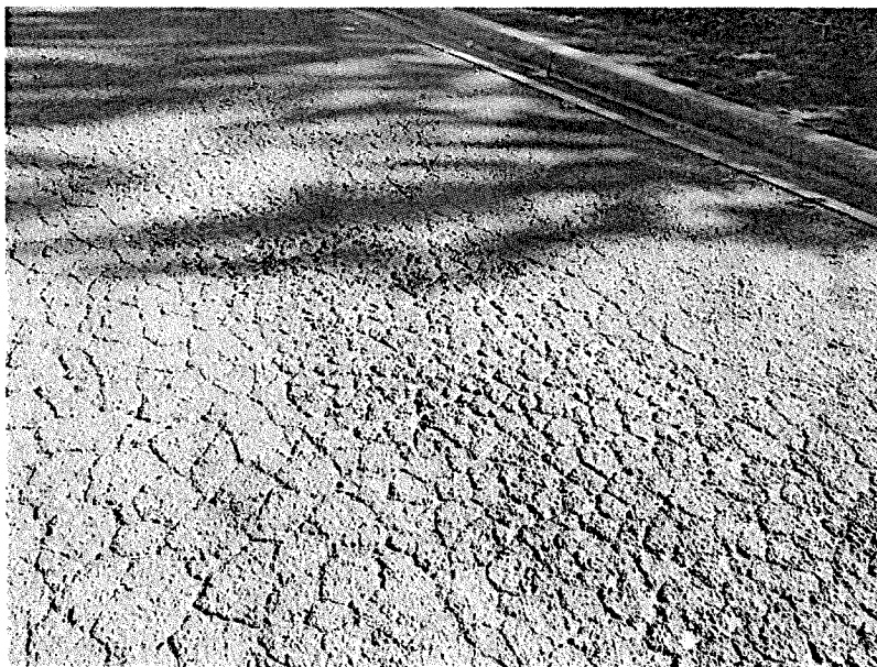
Figure 19: Pavement Condition - S.E. Falbo Drive
