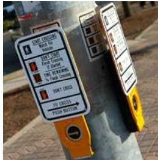
Figure 2.11 Accessible Pedestrian Signal and Pushbutton example (WSDOT)
