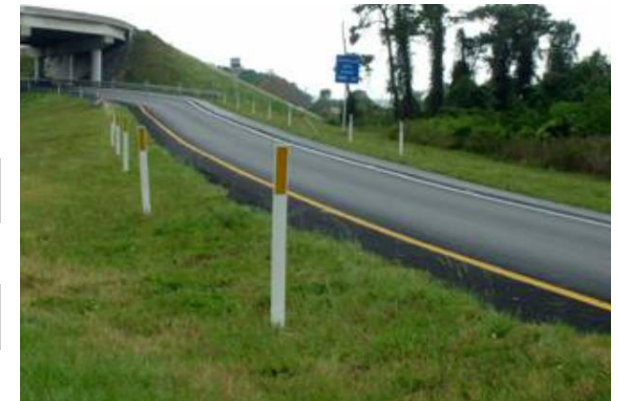
Figure 38: Roadway delineators installed on a ramp; image source: FHWA
