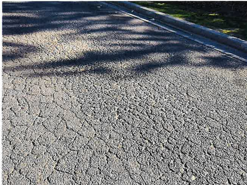
Figure 19: Pavement Condition - S.E. Falbo Drive
