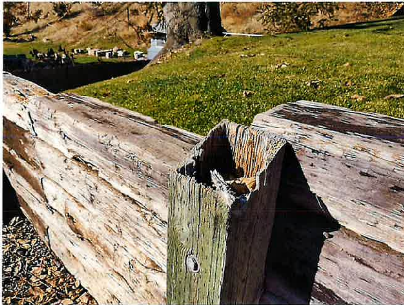
Figure 8: Retaining Wall Post Condition
