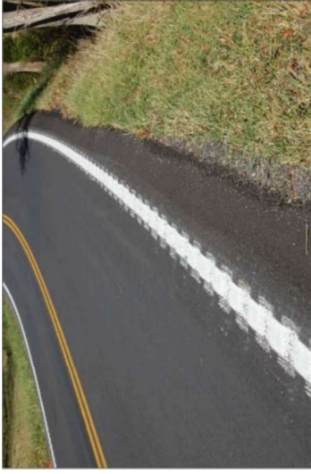
Figure 39: Edge line rumble strips along a roadway; image source: KYTC
