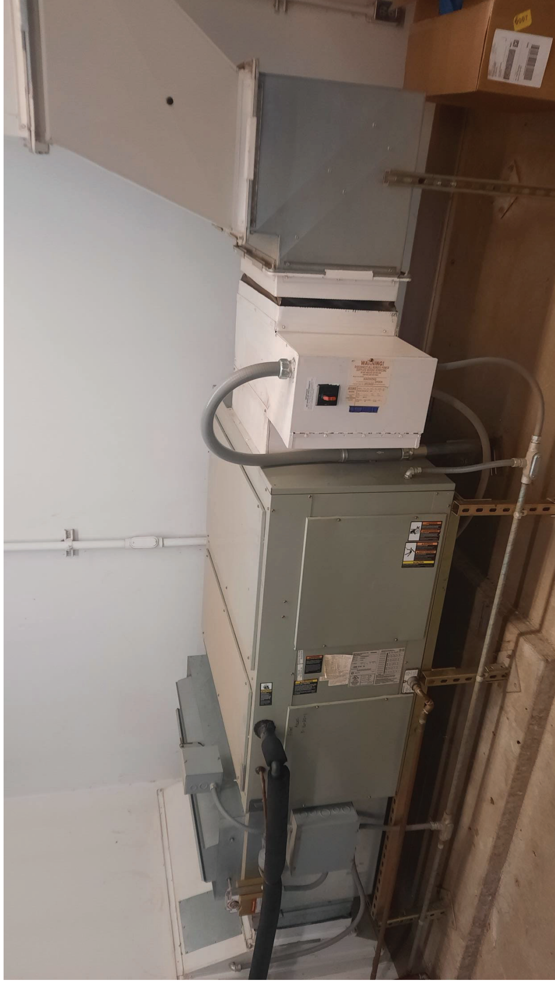
Air Handler with In Duct Heating Elements
