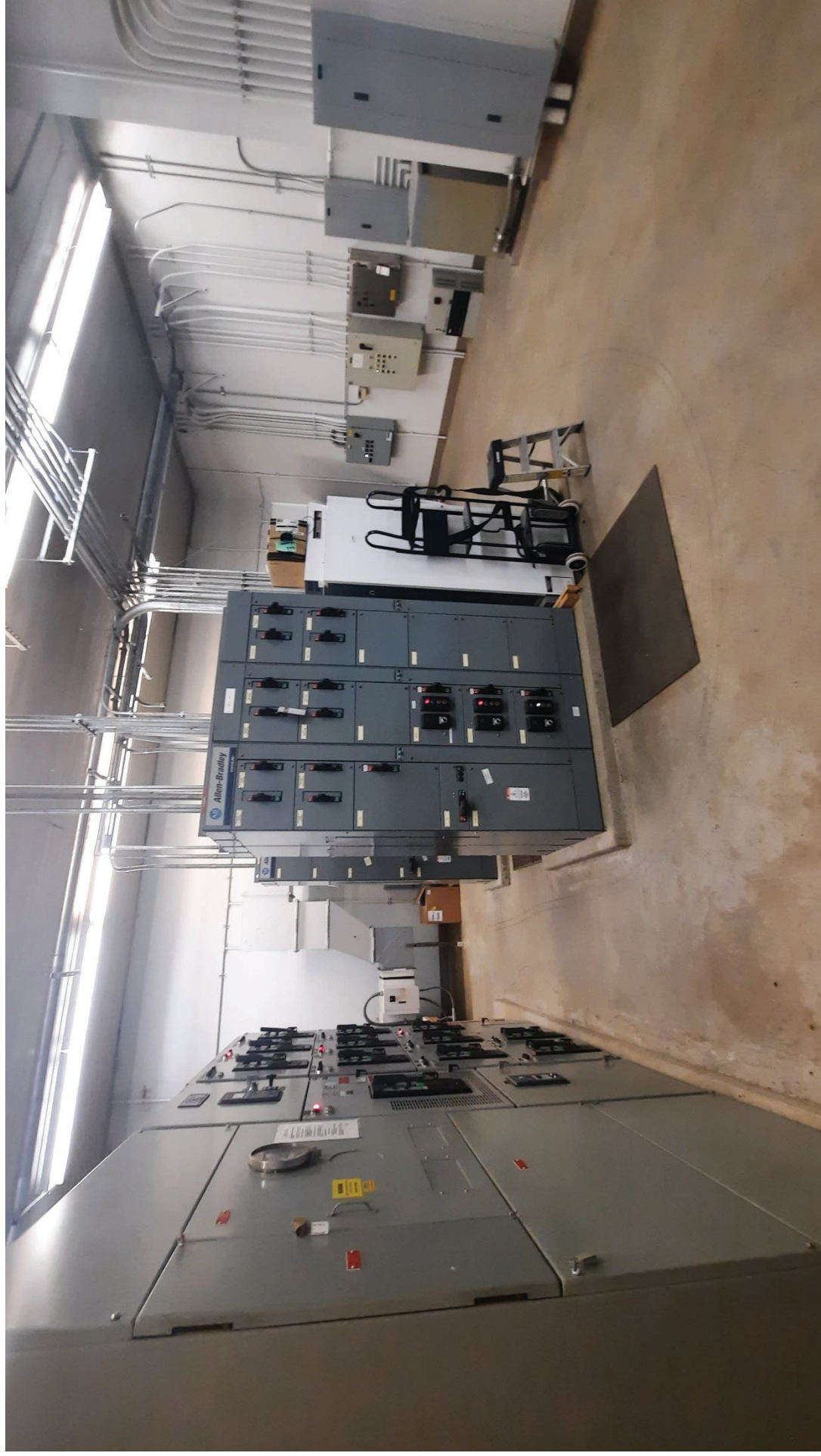
Treatment Building Electrical Room
