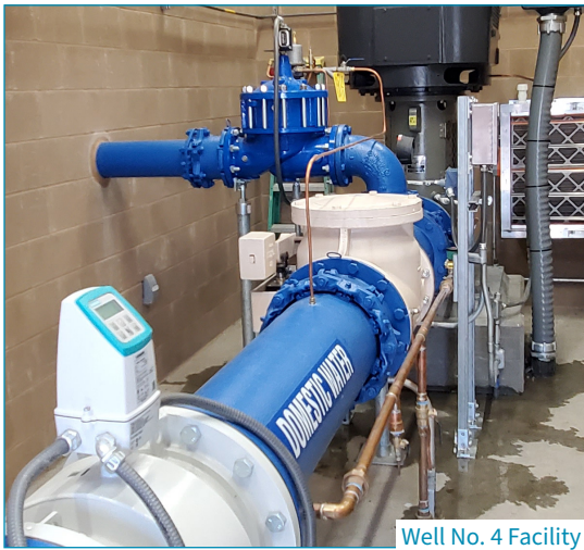
Well No. 4 Facility
