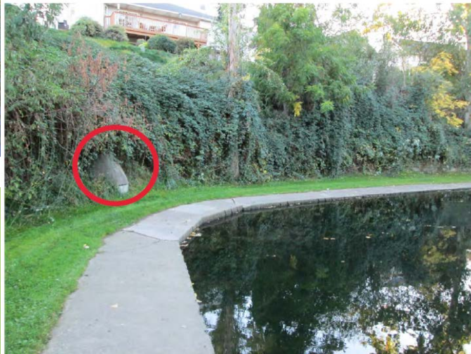
Photo 5. Stormwater inlet pipe to the fishing pond.
