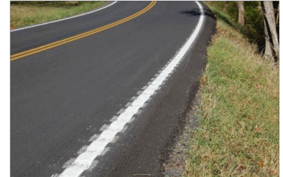
Figure 39: Edge line rumble strips along a roadway; image source: KYTC
