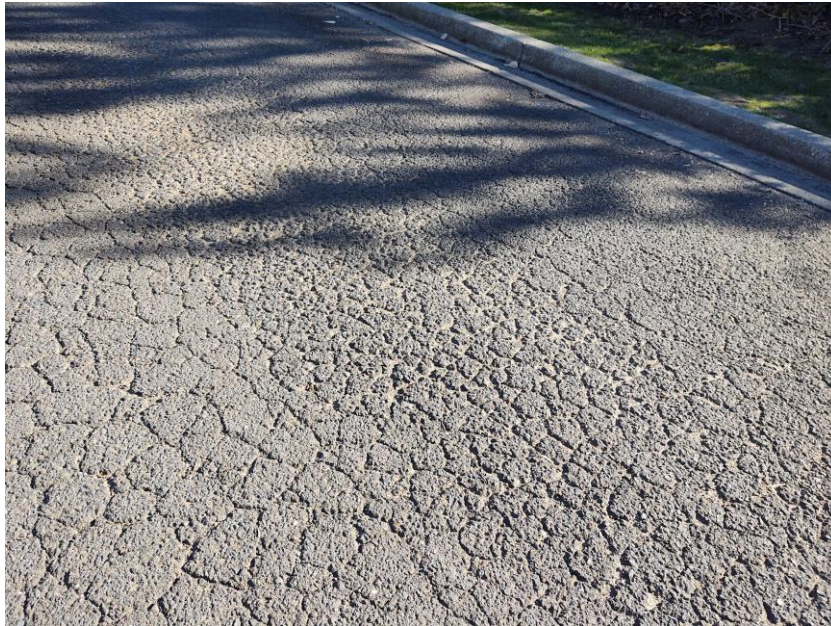
Figure 19: Pavement Condition - S.E. Falbo Drive
